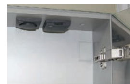
Detail - el. socket + switch Berker placed inside R ZS, PIR ZS
